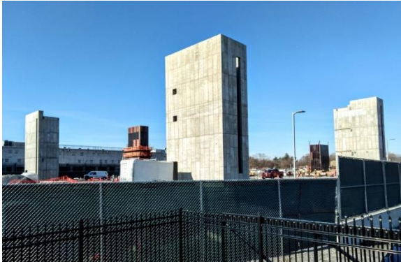
Dutchess Co. New Justice & Transition Center under construction (Image courtesy of the MidHudson News online)
